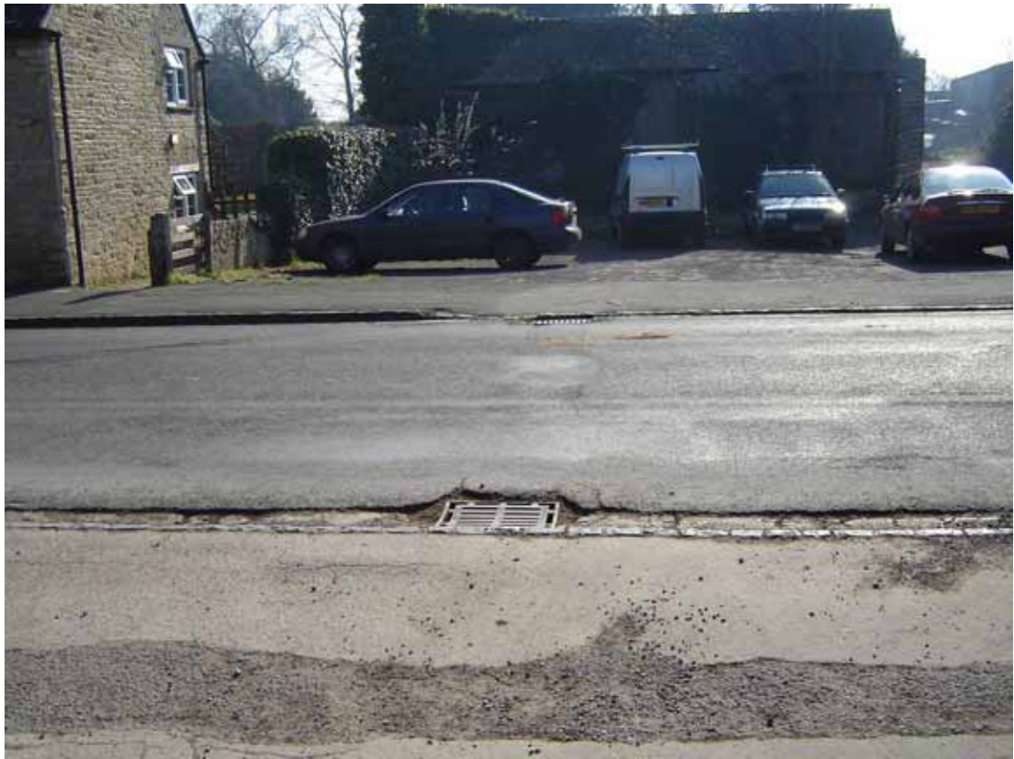
Area 1 - Gullies in low area of Blackditch Road
