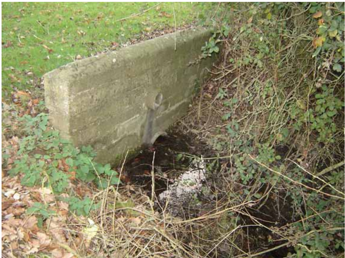
Area 2 - Sutton Pond Pipework Outlet
