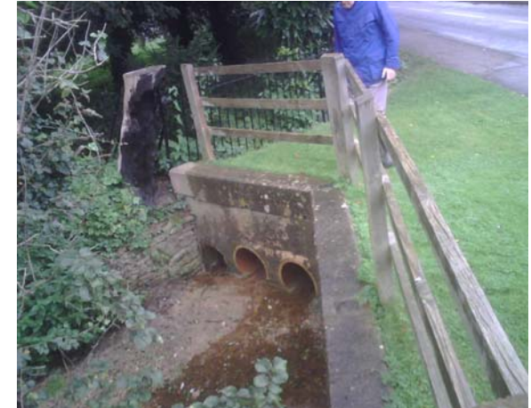
Area 2- Highway drainage culvert opposite Foxwell Court. Culverts pass under Yarnton Road. They convey water from enmained Elms Road ditch. Note: Sediment and debris blocking grated culvert
