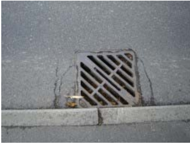
Area 2- Water damage around gulley outside Foxwell Court
