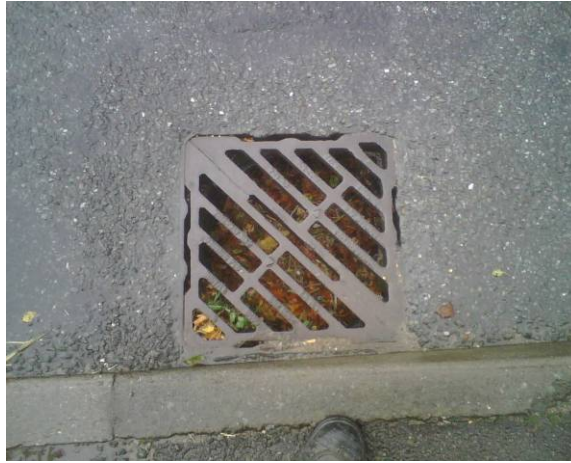
Area 2 - Blocked grating on Yarnton Road, near Foxwell Close
