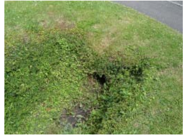
Area 2- Highway drainage opposite Foxwell Court
