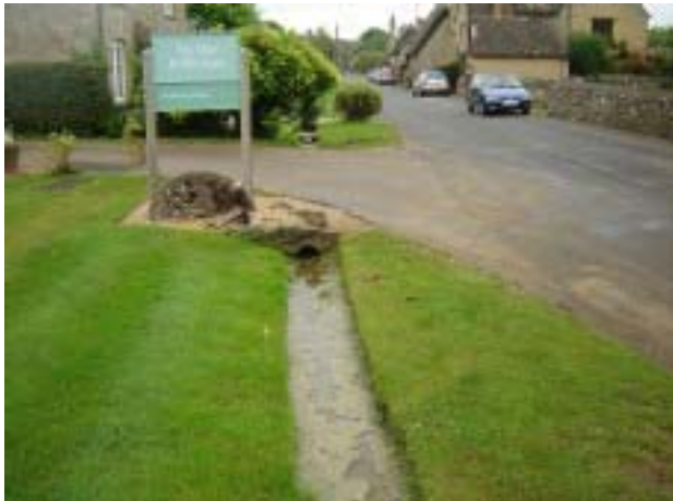
Area 2- Flooded ditch, Frontage of properties'
