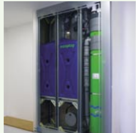
Rainwater harvesting system
