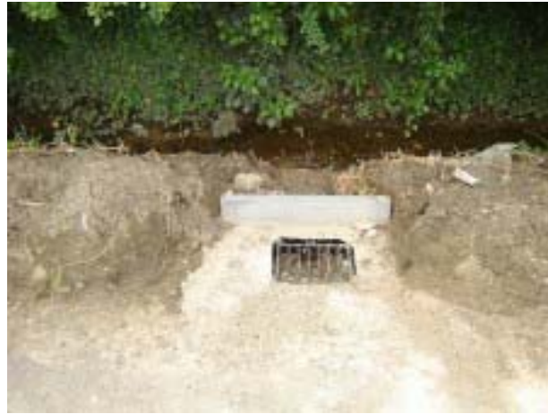
Area 1- Poorly constructed gully
