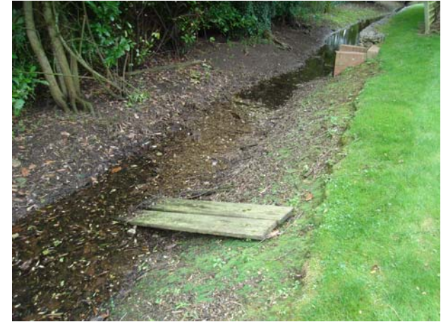
Area 3 – ditch obstruction behind flats
