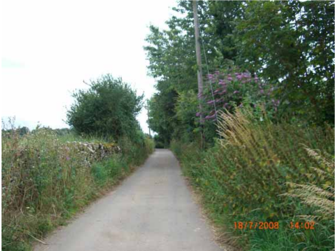
View north along Greenwich Lane. Dry stone wall (left of picture) and grass verge (right of picture) prevent surface water from exiting lane. No evidence of highway drainage (gullies).
