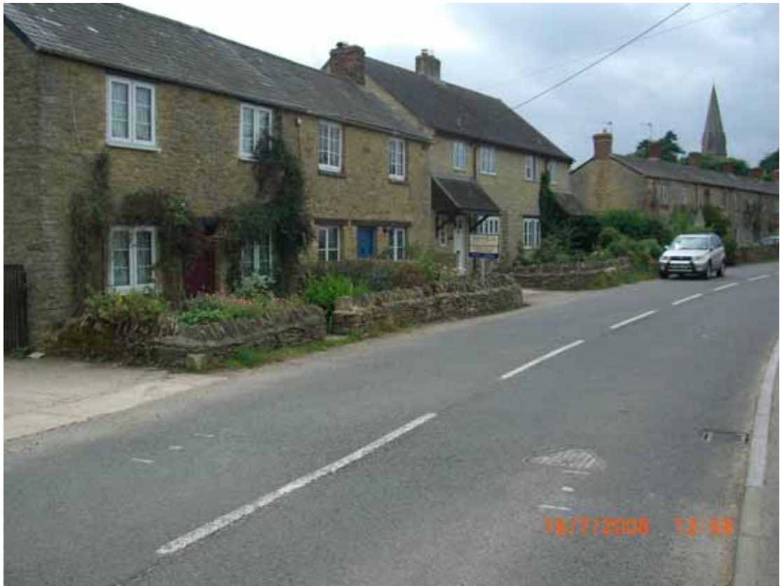
Two affected properties on Lower End in the foreground. Flooding caused by surface water run-off from highway.
