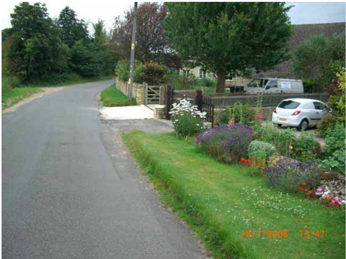
Affected properties on Buttermilk Lane. Mitigation measures have been implemented to property in distance (wall and linear drain).
