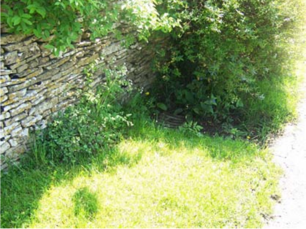
Photo 17: Drain at low point in Asthall Leigh
