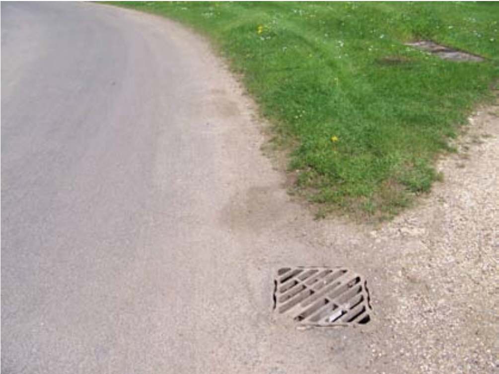
Photo 16: Gully pot located at the access road to Asthall Farm
