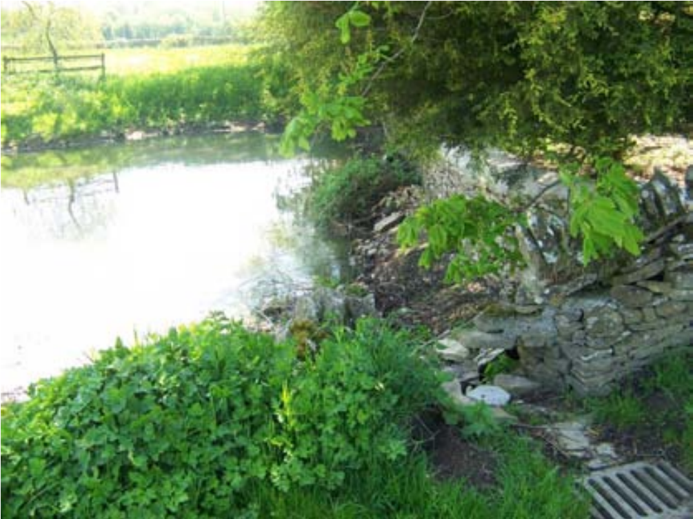
Photo 15: Collapsed wall by pond in Asthall, damaged due to flood waters
