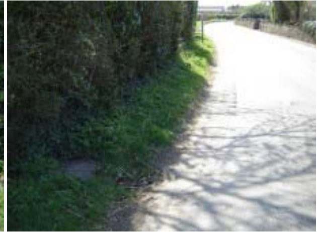
Blocked gullies outside Newman cottage, Broadwell (area 3)
