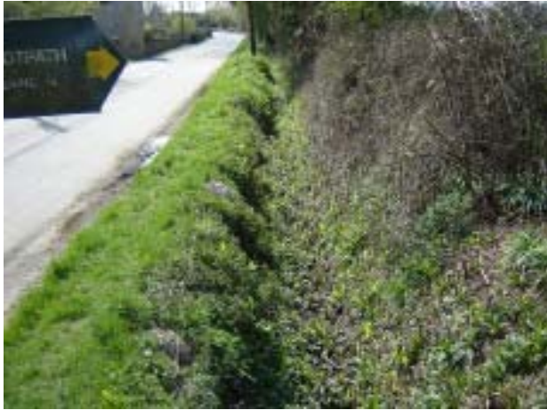
Ditch opposite Sunnyside, Broadwell (area 3)
