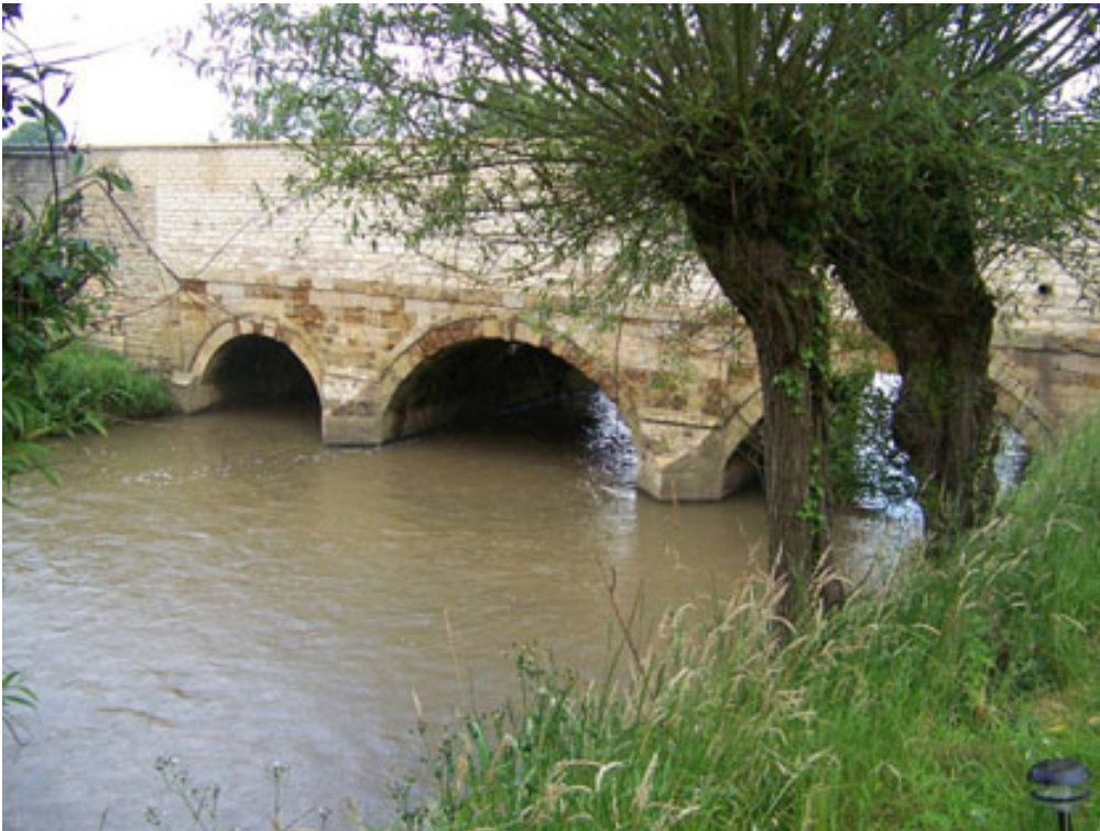
Looking upstream on the River Evenlode towards Dyer's Hill Bridge (taken July 2008). Prior to the flood event, one of the three arches was blocked. All three arches are now clear to allow flow to pass through. The parapet wall was damaged by the flood and this has now been rebuilt.
