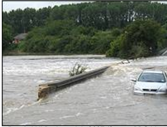
Flooding at Dyer's Hill Bridge in July 2007 (Source BBC News Website) The parapet wall on the left of the photograph has been damaged by the flood.
