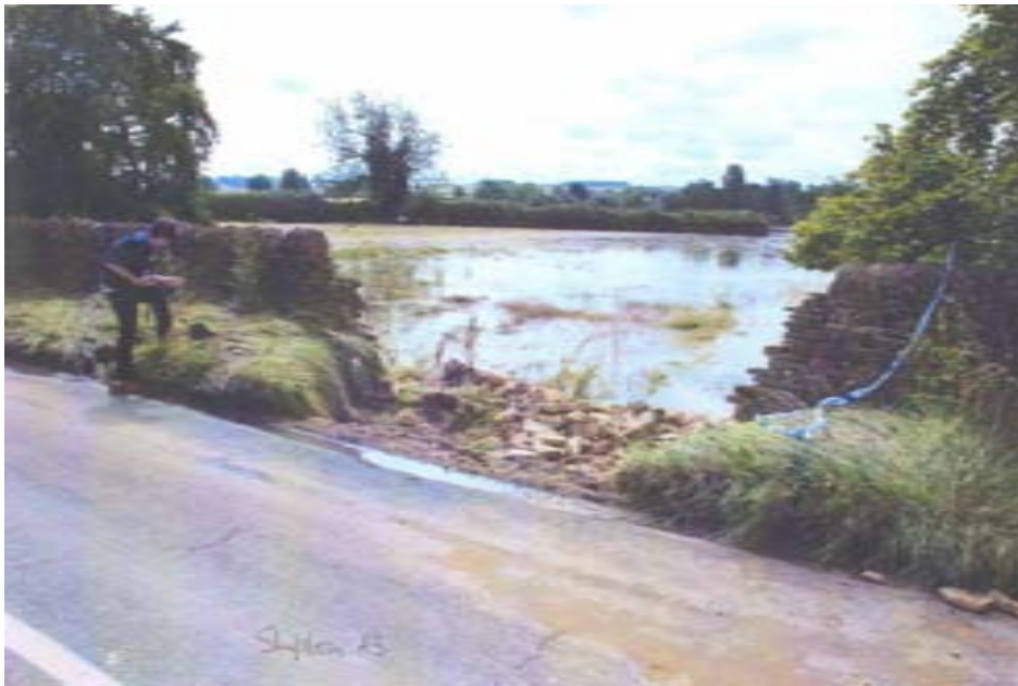
Damage to Station Road Bridge caused by flood waters from the River Evenlode
