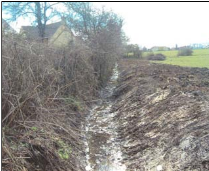
Cleared ditch behind Little Brook Meadow
