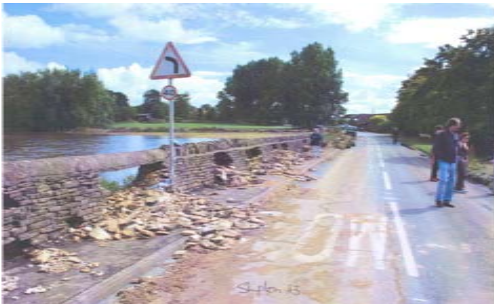
Damage caused to Station Road Bridge by floodwaters from the River Evenlode
