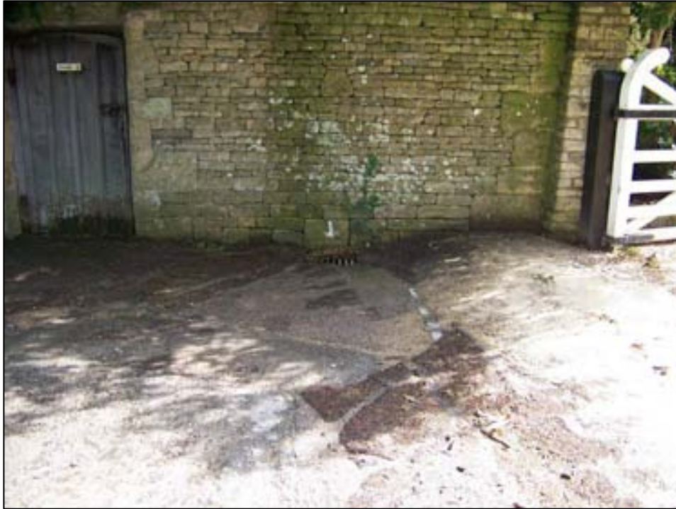
Gully located at end of Church Street at Prebendal Wall. Outfall location to be defined.
