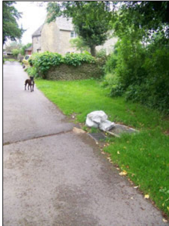
Photo 5 – Highway drainage gulley located at the end of Mill Lane, connects to the Shill Brook.
