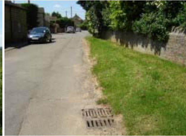
Area 2: Highway Drainage in Bull Street.
