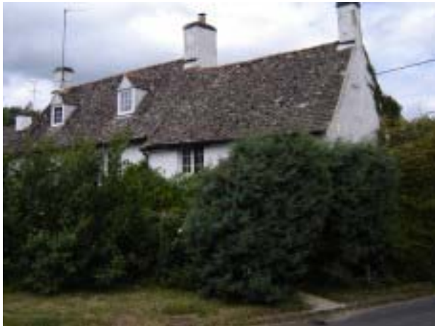
Area I - Flooded Property
