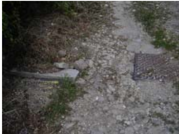
Area I - Highway drainage in Dark Lane
