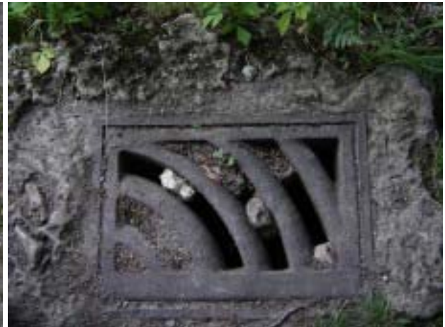
Area I - Highway drainage in Dark Lane
